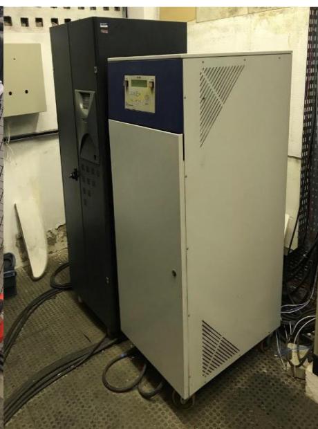
Figura 2 - UPS 1 e UPS 2
